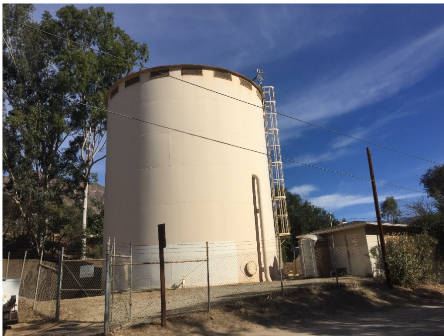
Photograph 6. View existing Arbolada tank within BSA, facing northeast (Unit B). Note ornamental vegetation surrounding the project footprint. November 13, 2018.
